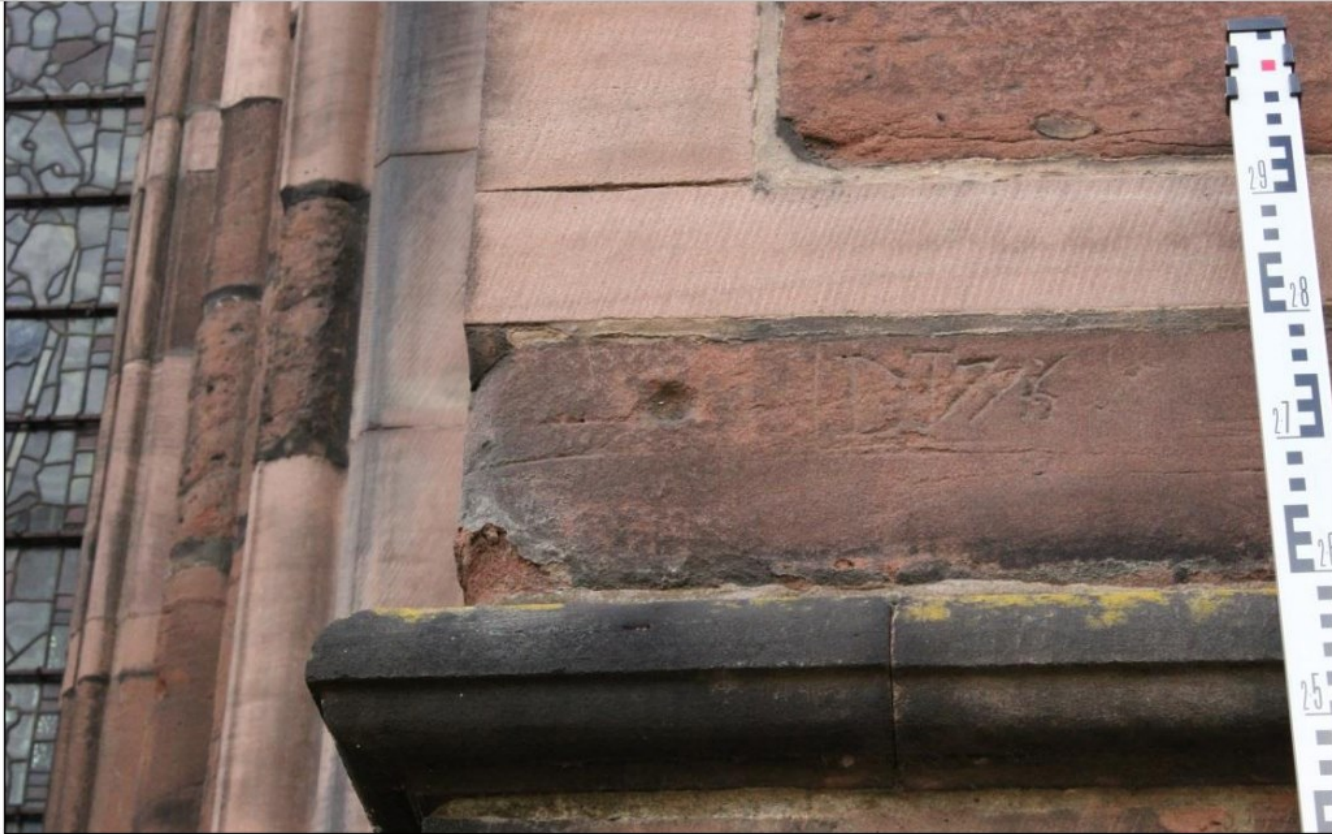
Figure 5: Photograph of stone replacement adjacent to an impact scar at Chester Cathedral
